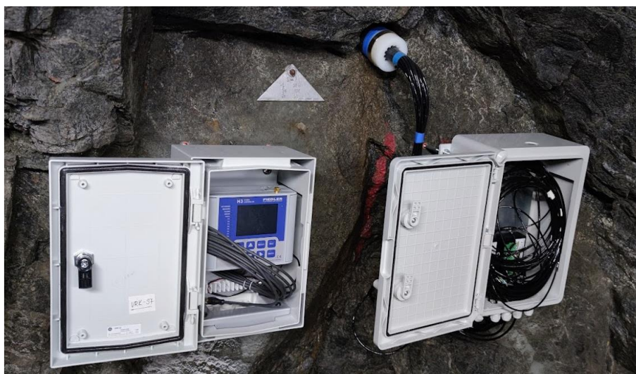
Fig. 25 – End of a monitoring borehole and the measurement equipment
