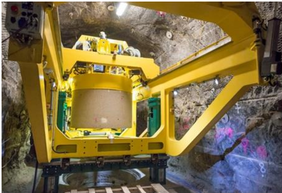
Figure 5-5. Posiva prototype buffer installation machine above a deposition hole (Figure Posiva). The assembly of the final version for operating is underway.
