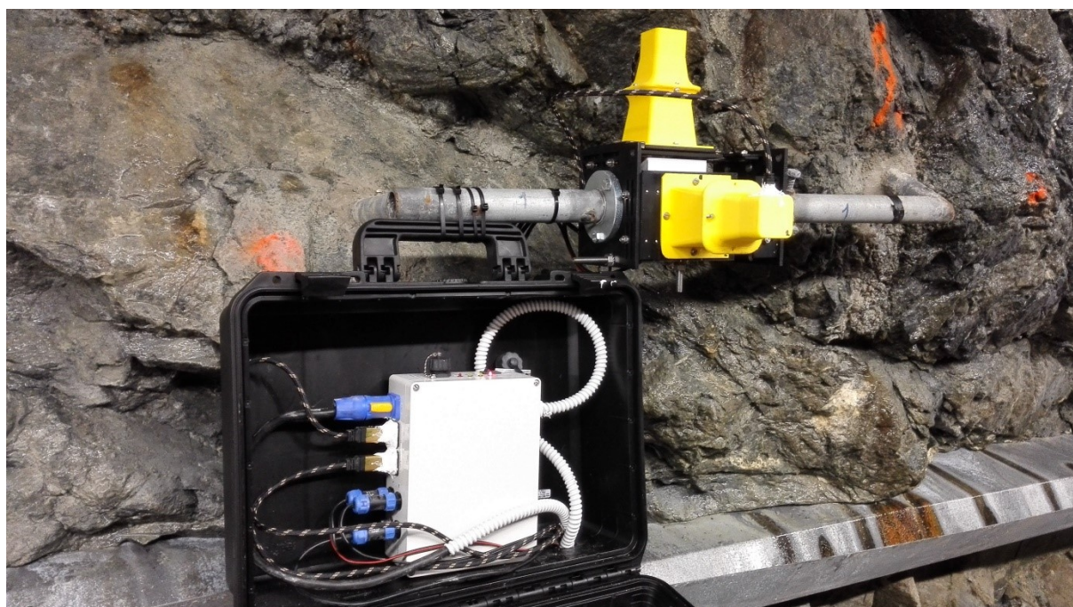
Fig. 1 Extensometer No. 296GWB0001 that is equipped by data-taker.
